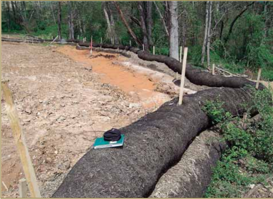
Compost sock sediment trap at Delta Ridge Residential Development in Delta, PA.
